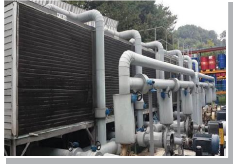
Cooling tower Facility View
