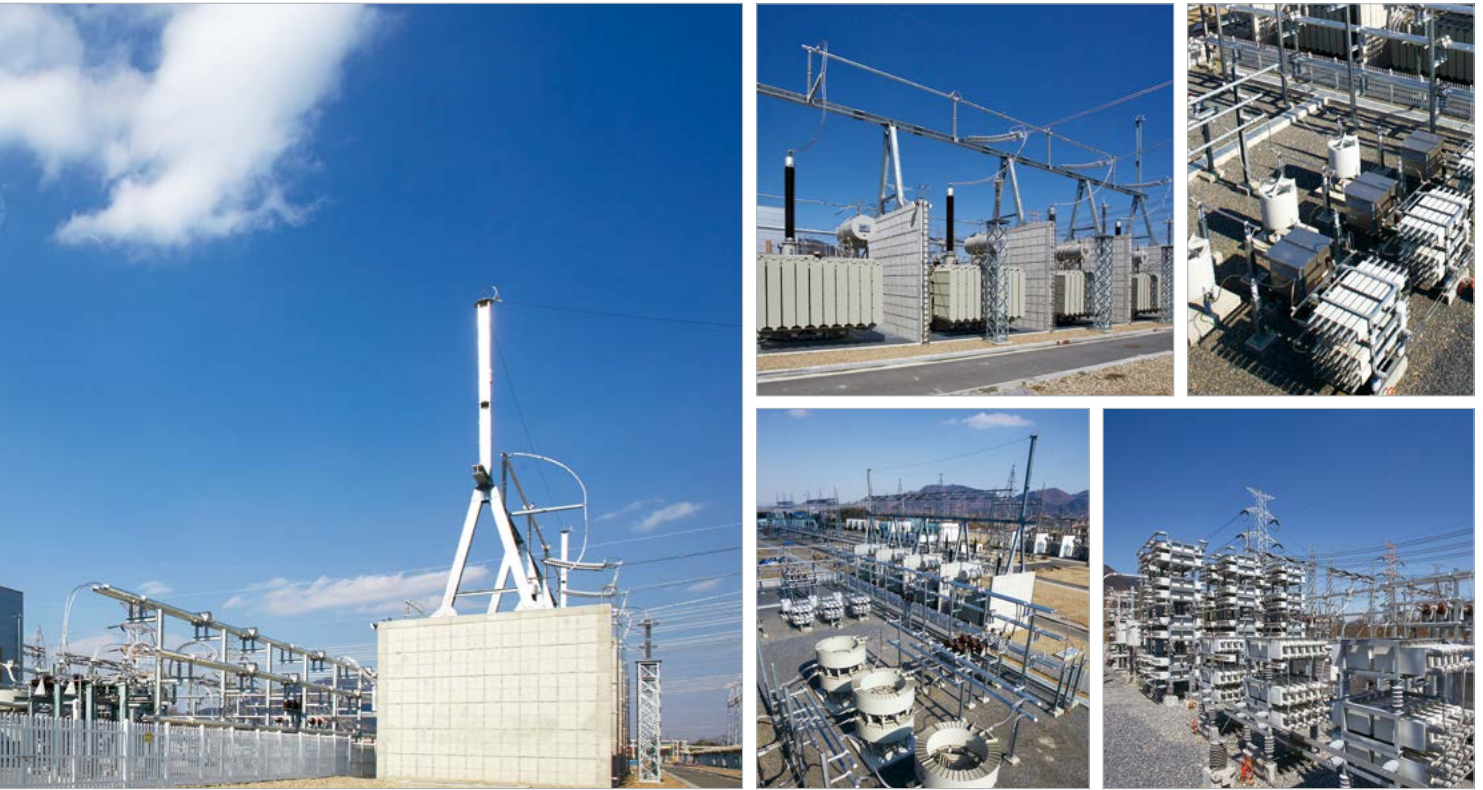
SVC, Korea(in KEPCO 345kV substation) TCR, TSC, AC Harmonic Filter (지상용량225 Mvar/ 진상용량675 Mvar) SVC 변전소
