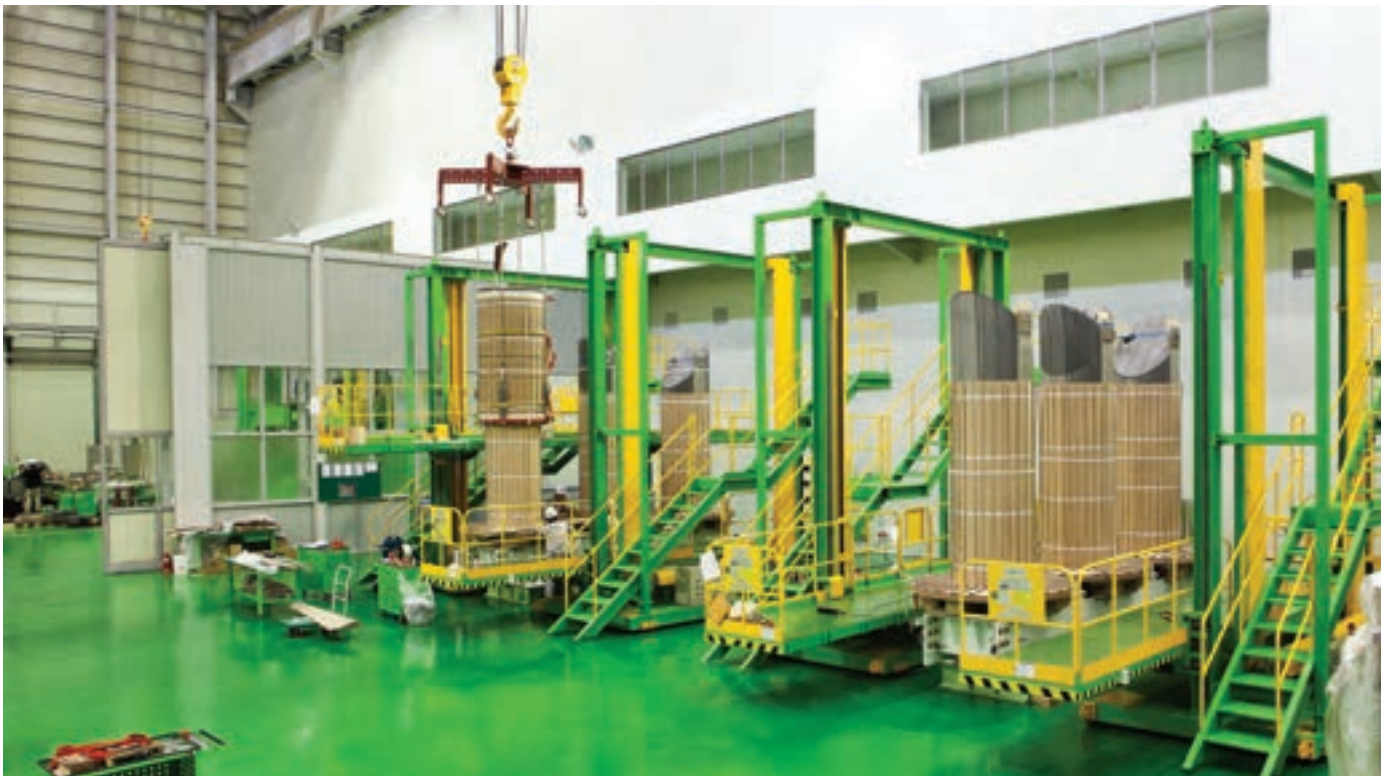
· CORE AND COIL ASSEMBLY SHOP
