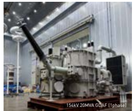
154kV 20MVA GDAF [1phase]
