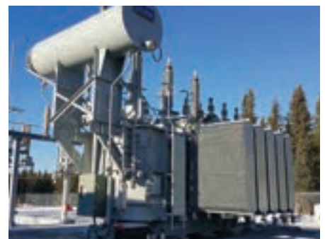
CANADA, 3 PHASE 138kV 42MVA
