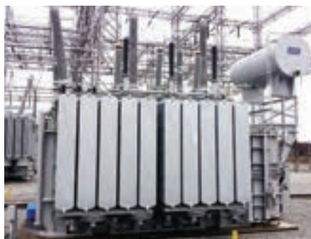
USA, 3 PHASE 345kV 448MVA
