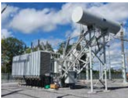
USA, 3 PHASE 500kV 350MVA
