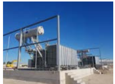
Australia, 3 PHASE 132kV 45MVA
