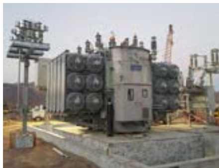
USA, 3 PHASE 69kV 150MVA
