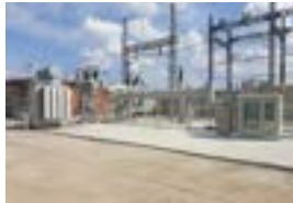
72.5kV GIS Outdoor substation
