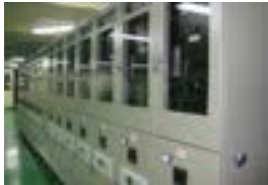
25.8/36kV GIS indoor Substation
