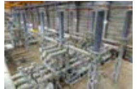
362kV GIS Outdoor substation
