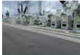
170kV GIS Outdoor substation
