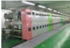
25.8kV E-GIS indoor substation
