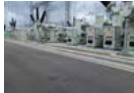
170kV GIS Outdoor substation
