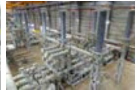
362kV GIS Outdoor substation
